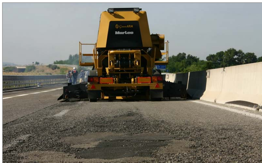
Figure 8. Raveling and Patching before AR2000
